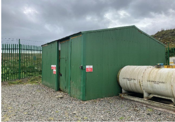
Evac area, ventilation unit and generators @ Evac site
